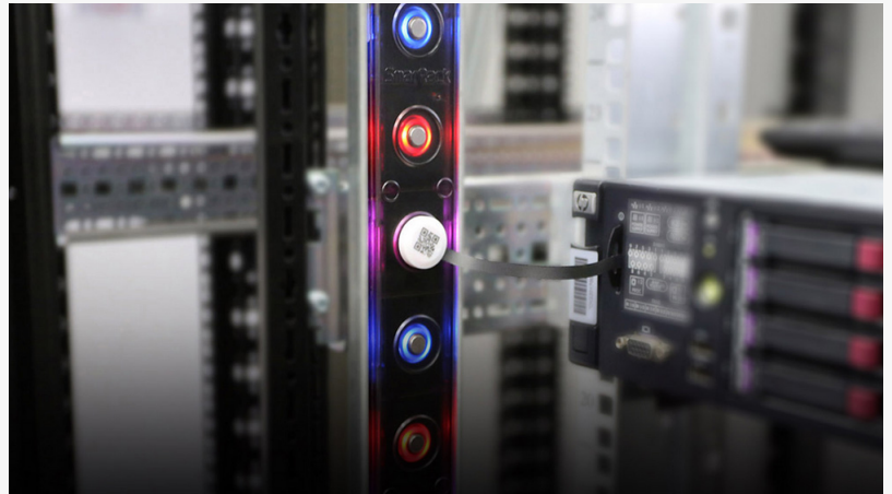
Digitalor's RFID asset tracking technology as shown in a data center rack.
