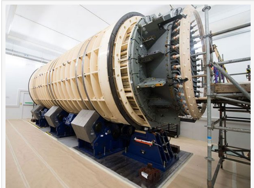
Siemens Energy customer DRAX Power in the UK a Power Roller System for a Parsons 660MW Generator.
