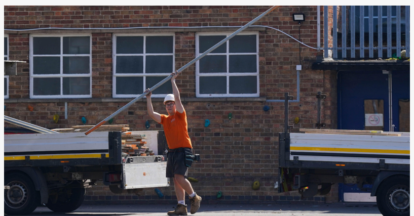
Remedial work being carried out at Mayflower Primary School in Leicester, which has been affected with sub standard reinforced autoclaved aerated concrete (RAAC). Picture date: Monday September 4, 2023. Source: Alamy / PA
