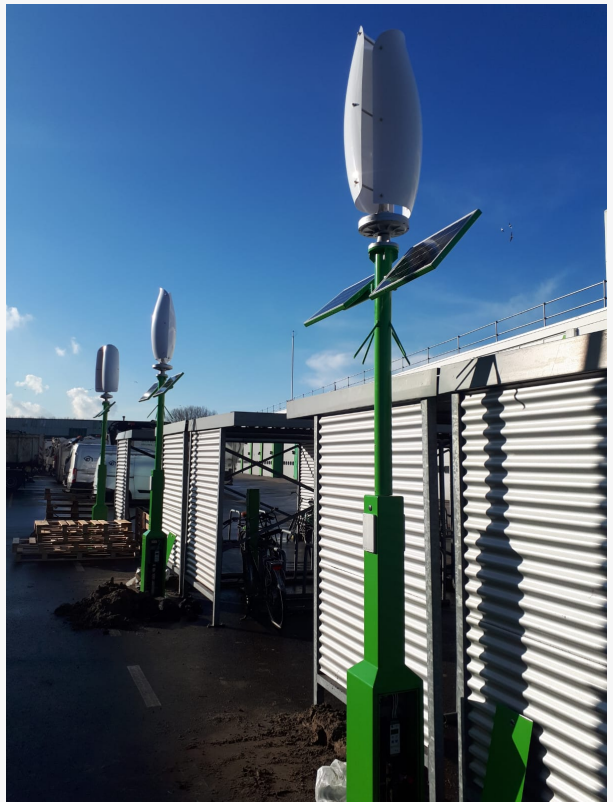
Wind and Solar E-bike Charging Poles
