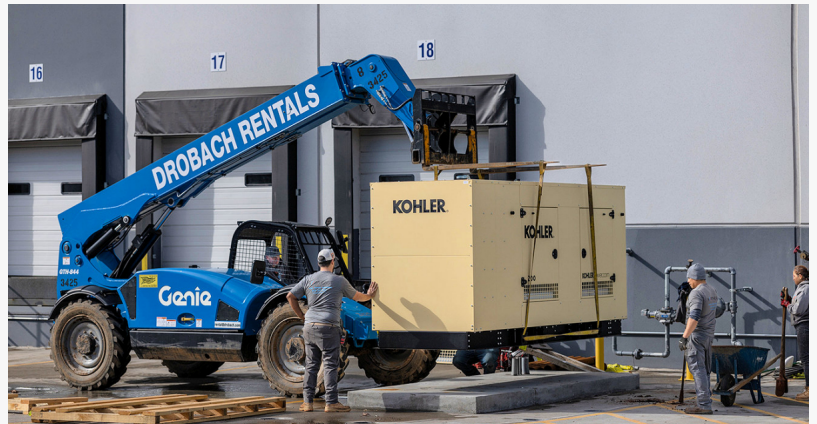
Northeast Generators has expanded its industrial generator services throughout New Jersey
