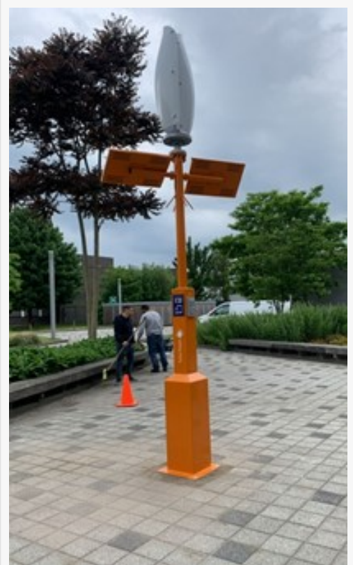
ZW Charging Station in Tilburg
