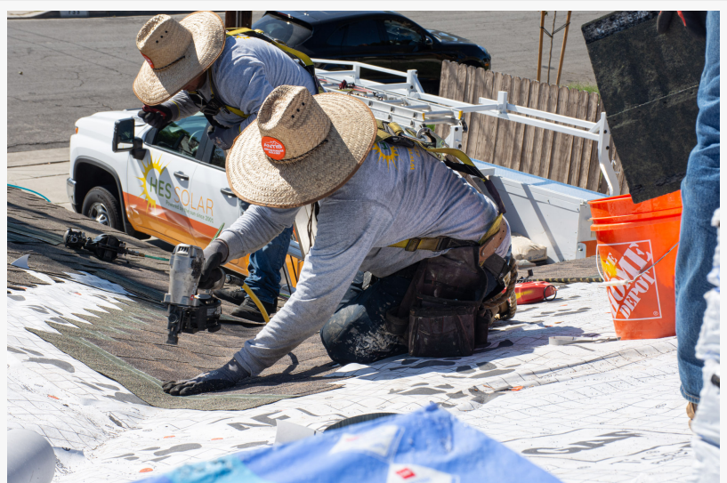
HES Solar's roofing crew is already installing new roofs on homes in San Diego County
