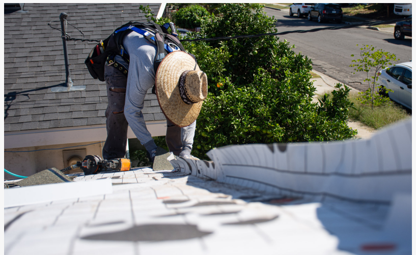
An HES Solar roofer works on a new roof installation after putting down fresh roofing paper.
