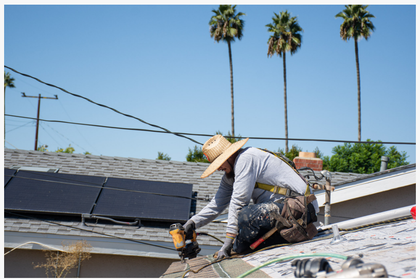
HES Solar's new roofing department is already up to speed and installing new rooftops in Southern California.
