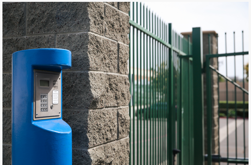
I-5 Self Storage Access Control Equipment.
