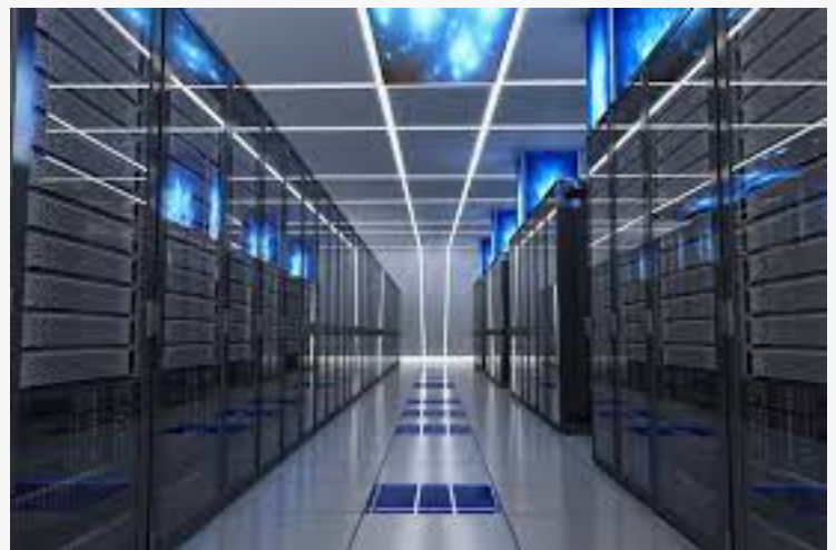
Data Center Power Market
