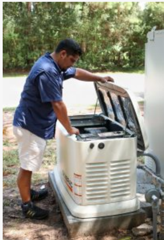
US Power Pros electrician working on a Generac generator
