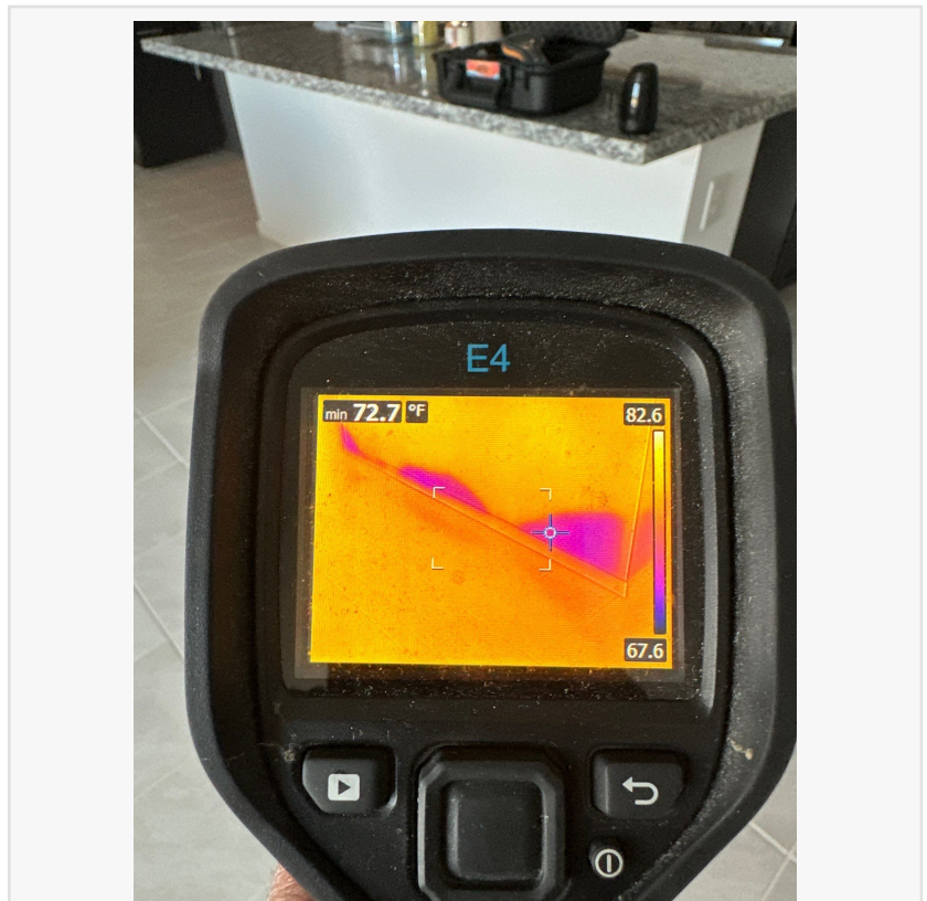
Thermal imaging showing hidden moisture in a kitchen island.
