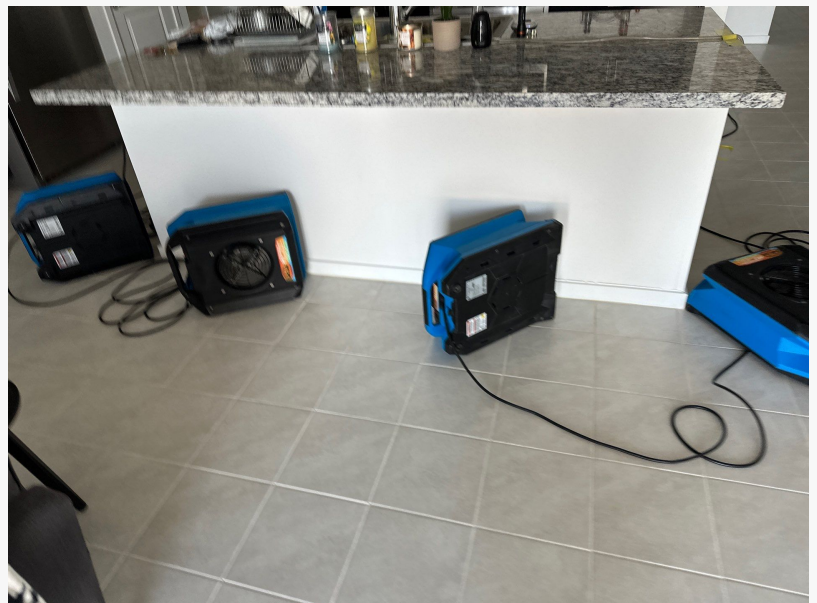
After finding the hidden moisture in the kitchen island, equipment was set up to dry out the damage.
