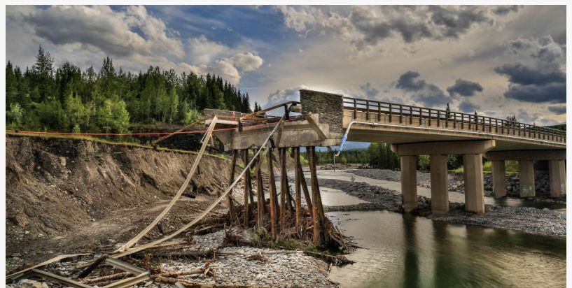
Previous flooding in Calgary, Canada destroyed a high way bridge that has yet to be repaired.
