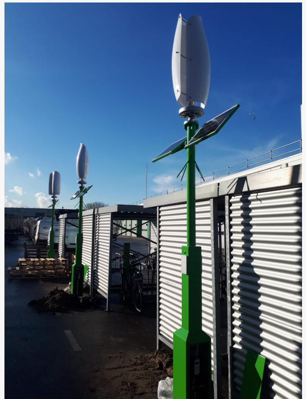
Wind and Solar E-bike Charging Poles
