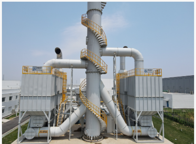
Leading the Way to Cleaner Skies: A glimpse of Ship & Shore China's latest air pollution control system installation, showcasing our commitment to a greener future.
