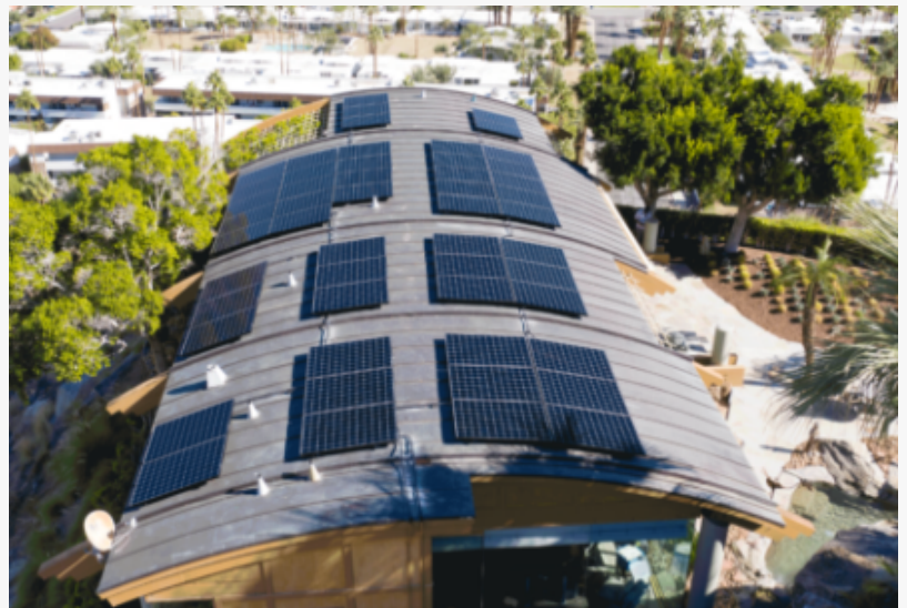
Renova Energy Residential Installation
