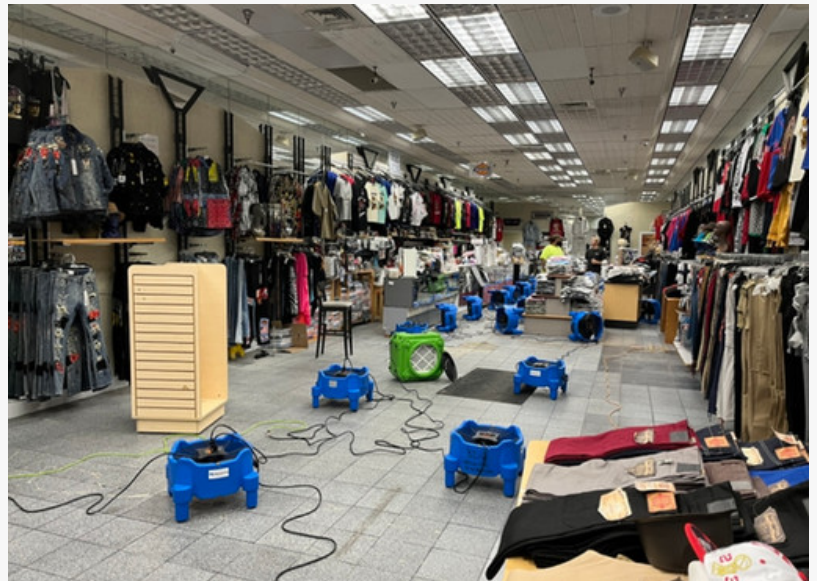
Fire damage restoration
