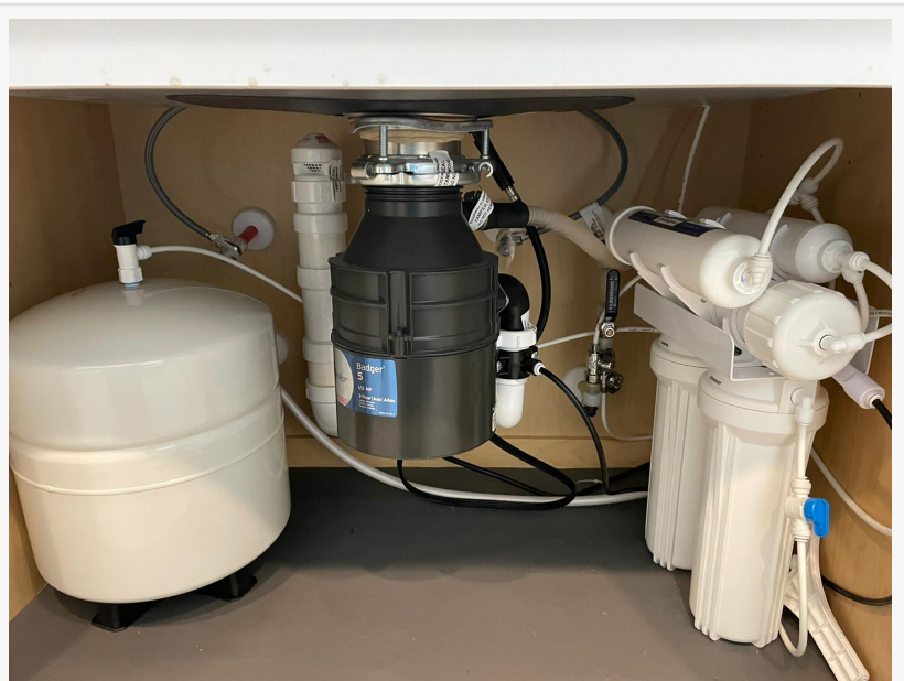
Reverse Osmosis in Port St Lucie
