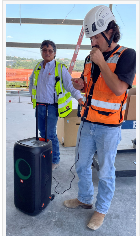
Joseph Sanderson a Project Manager at BCS Concrete Structures at the Nutrabolt project.
