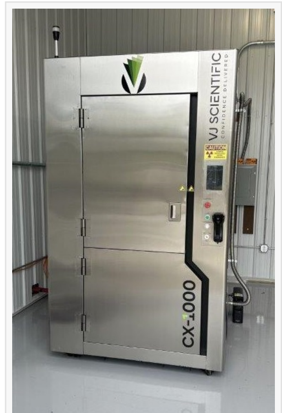
CX-1000 Cannabis Decontamination System Installed at Ohio Cannabis Facility
