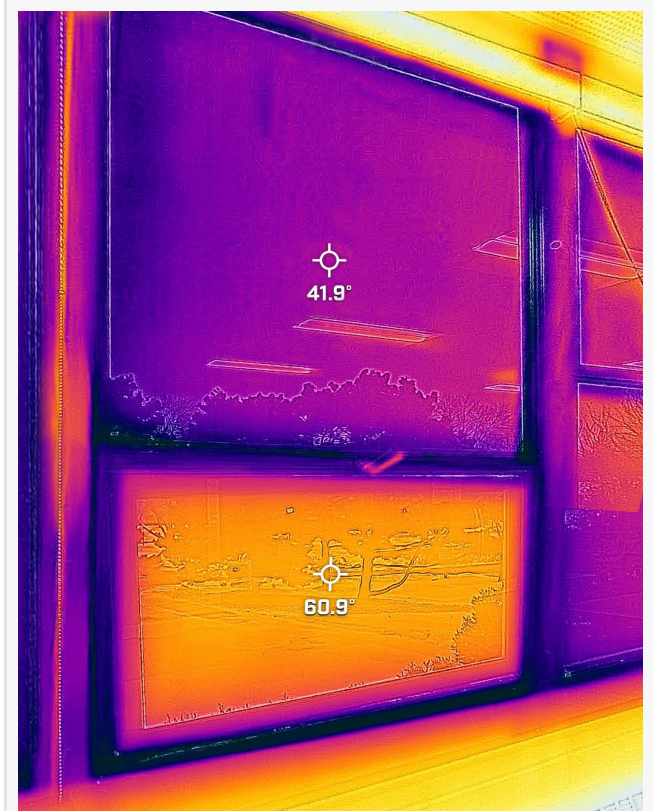
Infrared IR imaging shows 19°F difference between the retrofitted window on the bottom and the colder original window on the top, demonstrating it is significantly better at reducing heat loss. Photo by INOVUES.
