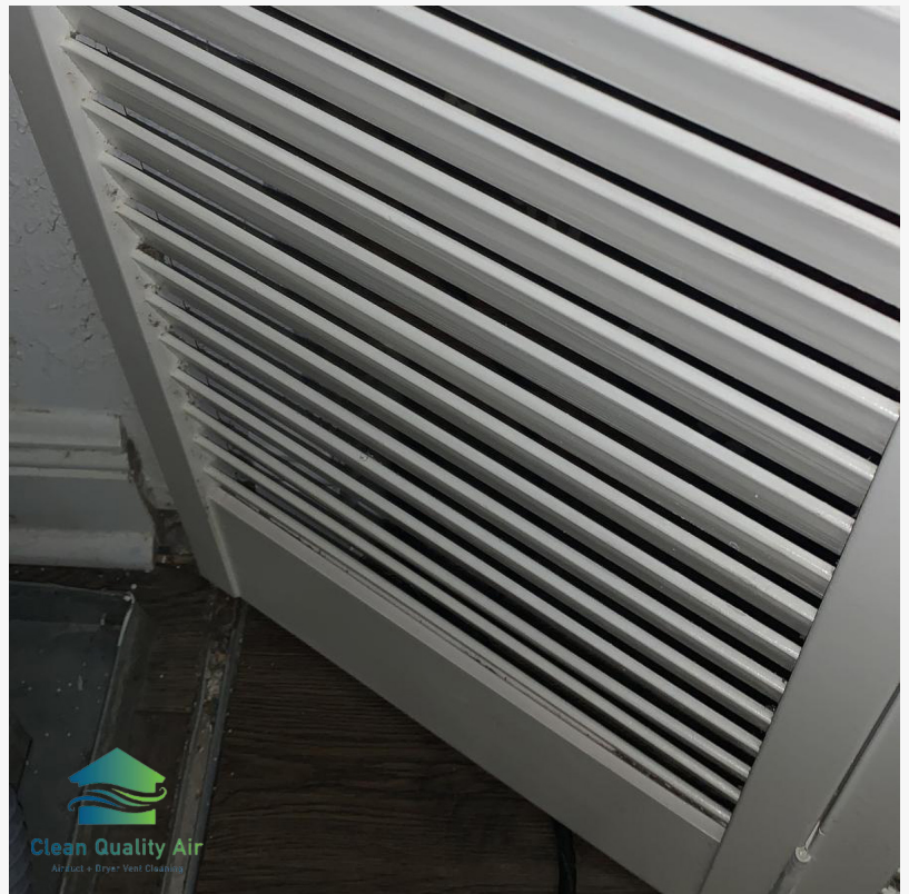
Air Duct Cleaning Services in Vero Beach
