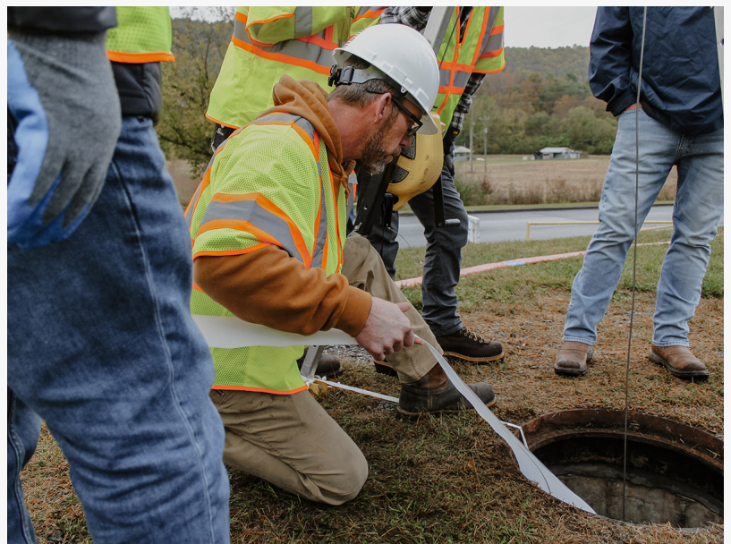
East Coast Infrastructure Team Performing Proper Installation Preparation Steps During Hands-On Training at Reline America Facility
