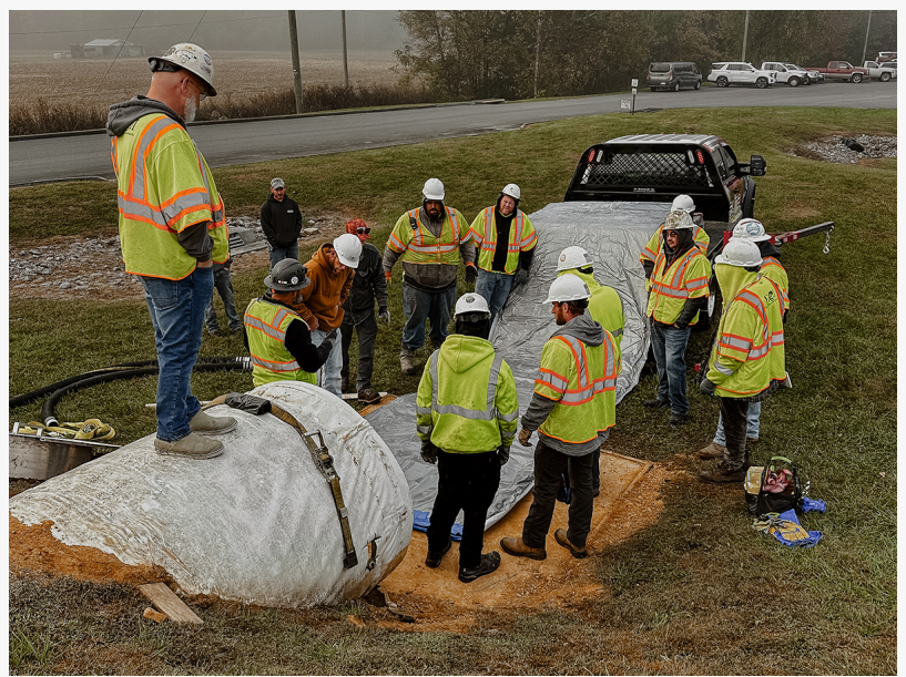
East Coast Infrastructure Team Participates in Hands-On Training at Reline America Facility
