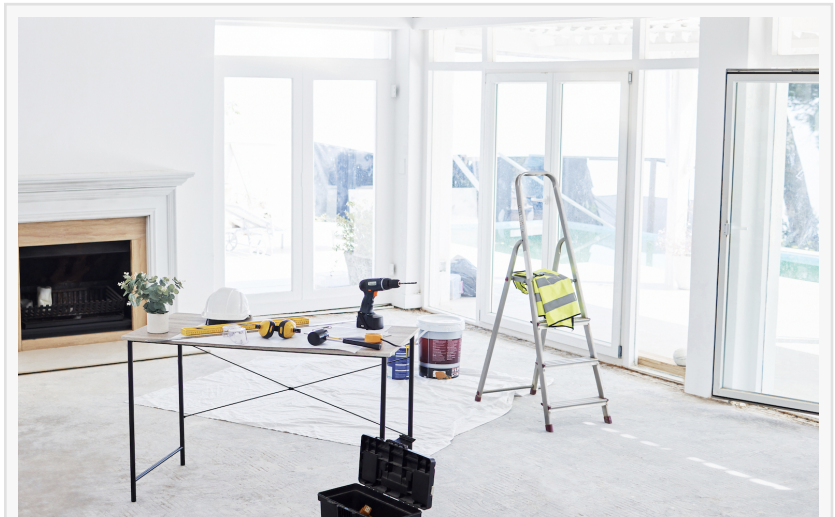
Room inside of a house under construction with tools, a fireplace, open windows, and a ladder.
