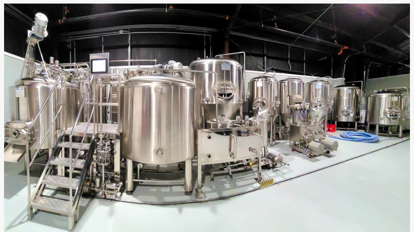
Turn 2 Brewery, built by MW Control Solutions
