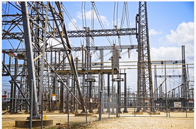
Texas Power Grid Substation. Image from Sam LaRussa for Unsplash.
