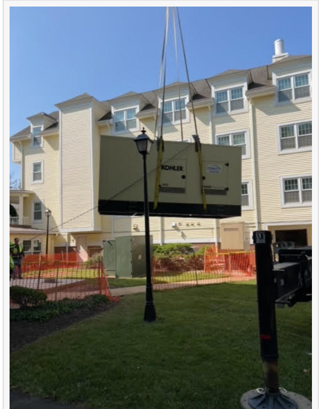
Large generator placement by DC Metro Commercial Construction team Scott-Long at Sunrise of Countyside Senior Living
