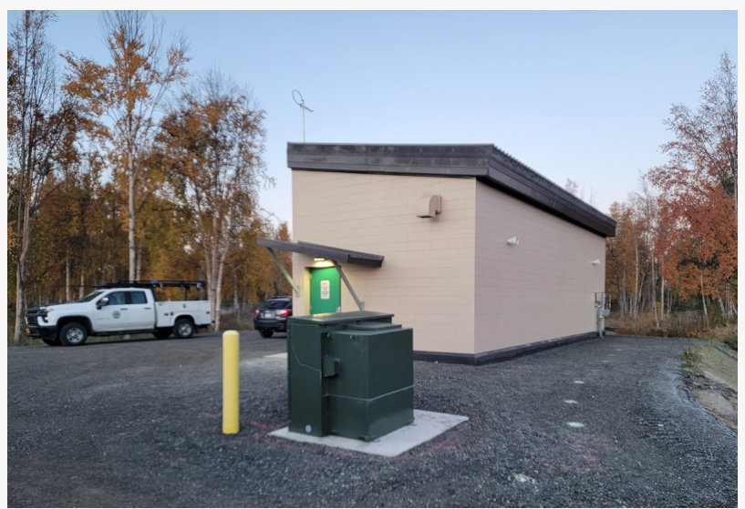
AWWU Pressure Reducing-Energy Recovery Station
