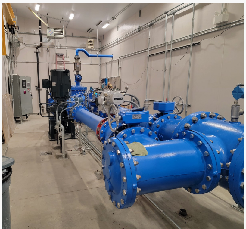
AWWU Flow-to-Wire Configuration
