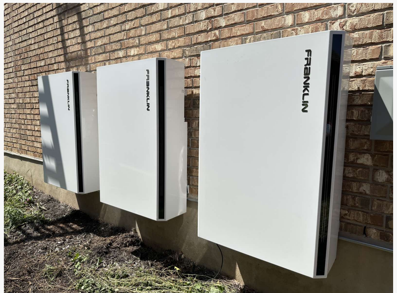
Franklin WH Batteries installed in the San Antonio area
