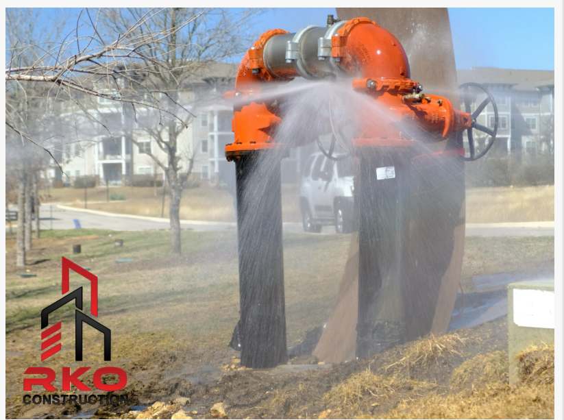
Burst pipe spraying water
