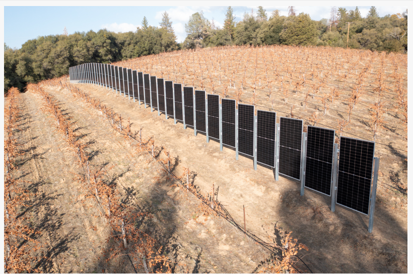
Sunzaun Installation on a Vineyard in Somerset, CA
