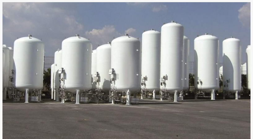
Cryogenic Tanks Market
