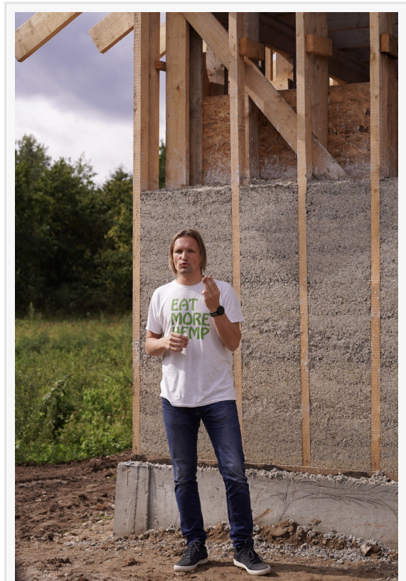
Sergiy Kovalenkov, Director of Hemp Technology, Ukraine, at the site of hempcrete accommodation construction near Lviv in western Ukraine
