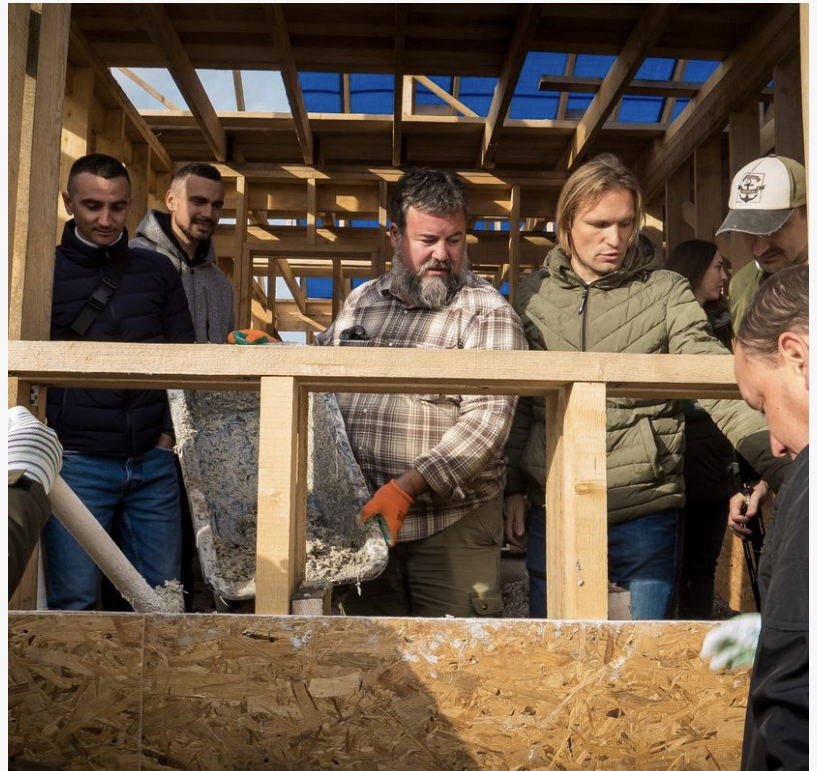
The Ukraine project team builds hempcrete housing in Ukraine for internally displaced people and war orphans
