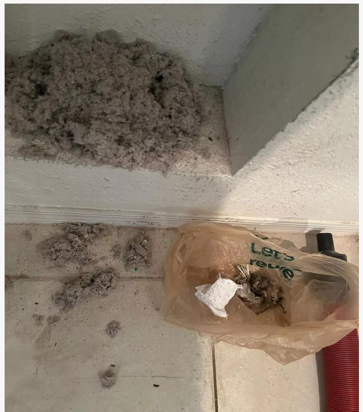
Air Duct Cleaning Port St Lucie
