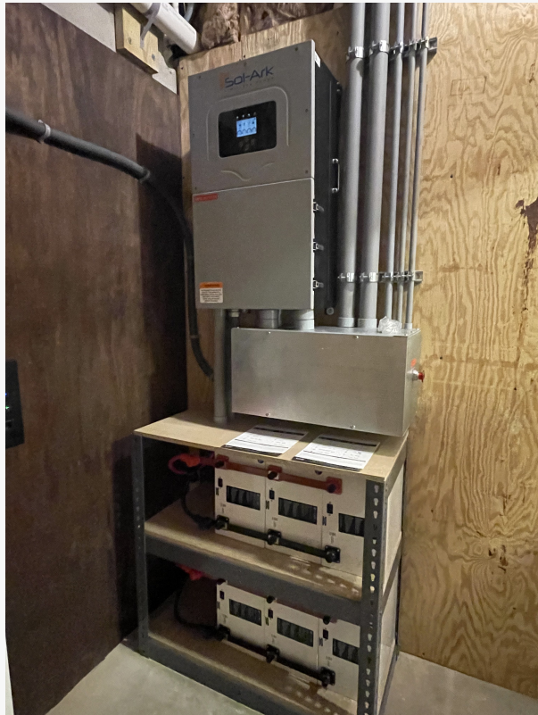
Sol-Ark inverter and SimpliPhi backup battery bank.
