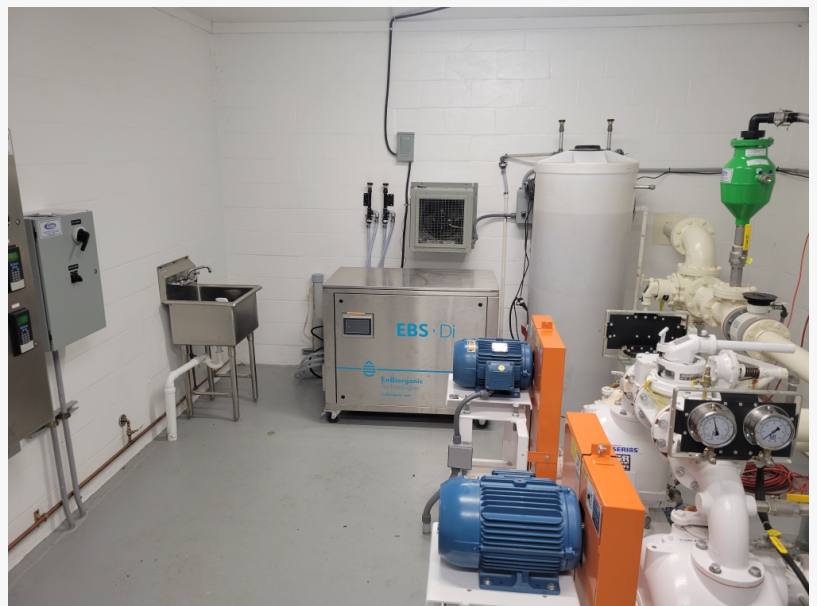
EBS-Di Installation at SSTA
