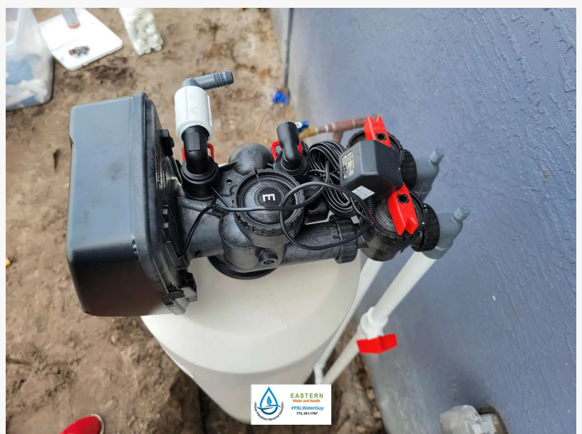
Reverse Osmosis Drinking Water For Yachts
