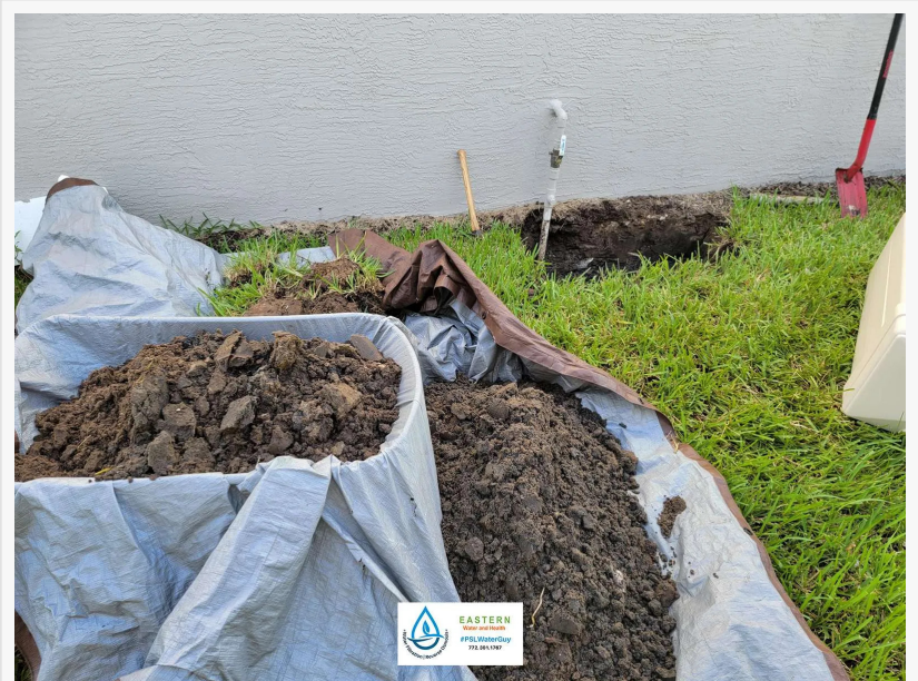
Residential Water Treatment In Port St Lucie
