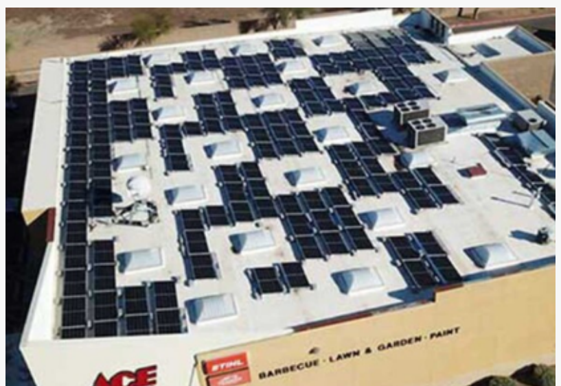
Arizona Solar Wave Commercial Installation
