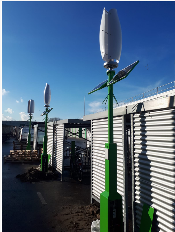
Wind and Solar E-bike Charging Poles
