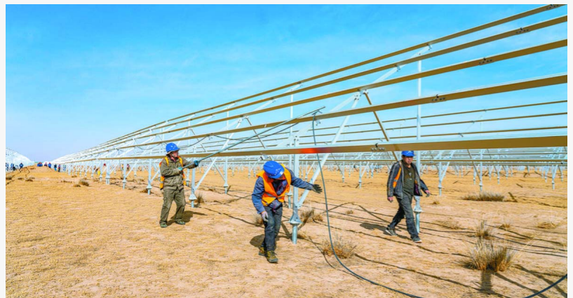
A common installation of PV panels on a PV project.
