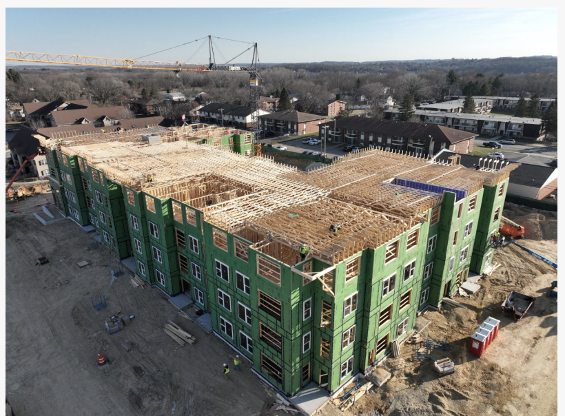
DC Materials provides quality supply and framing solutions for multifamily and commercial projects.
