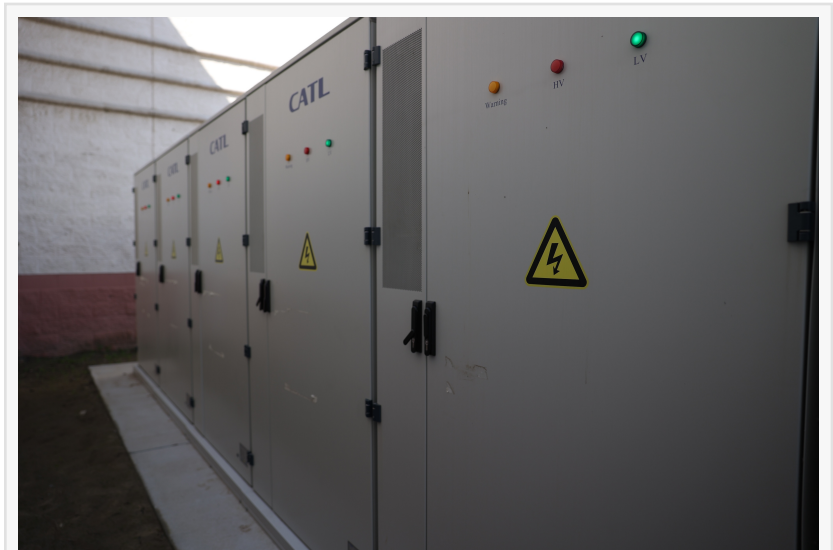
The 2 megawatt-hour Battery Energy Storage System will fully charge from a 2-megawatt solar system Blue Sky installed at Hanford Mall in Hanford, Calif.
