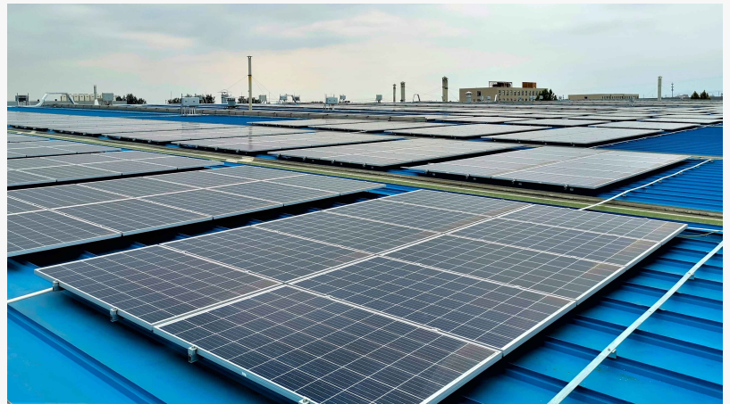
Solar panels on BWI Group's production base in Beijing, China, will cut 18,000 tons of carbon dioxide emission in total during 25-year period.
