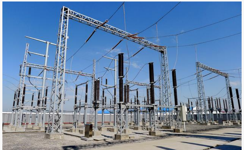
The main function of a substation is to convert the high-voltage electrical energy delivered to the substation into low-voltage electrical energy suitable for distribution or supply
