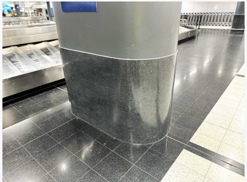
HANDCRAFTED: Terrazzo was troweled by hand on columns and existing terrazzo tiles were replicated with poured-in-place terrazzo in the new Terminal A at O'Hare Airport.
