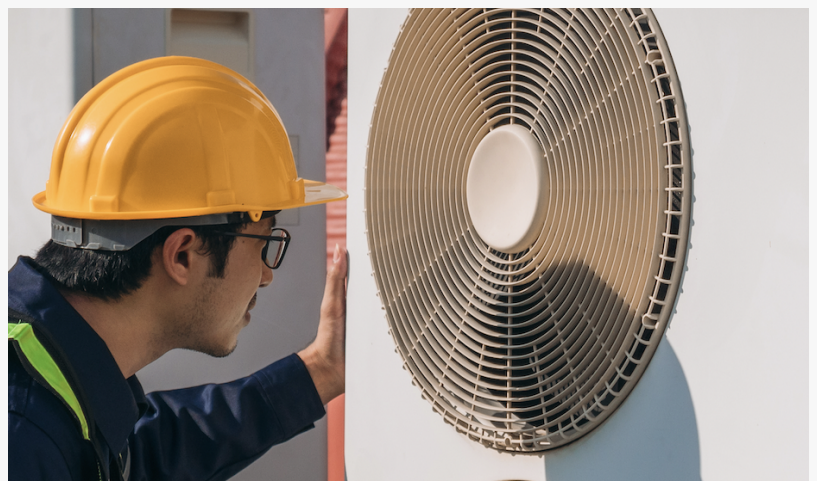
An aircon technician checks the building's air conditioning cooling system.
