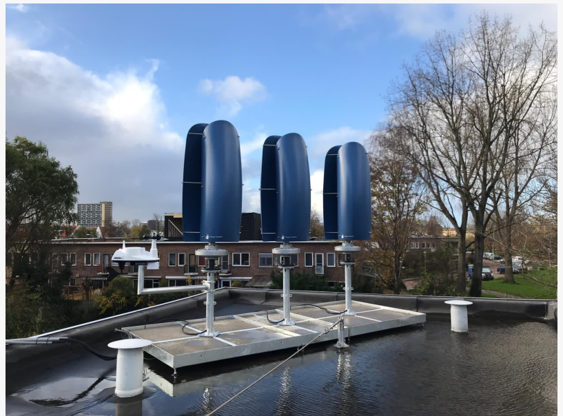
Three installed small size Wind Tulips
