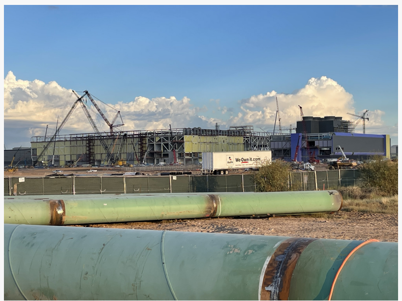
Certified AWS CWI inspectors from AWSCWI.COM documenting and evaluating a pipeline welding project.
