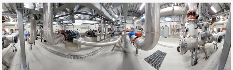
Rentricity's Dual Flow-to-Wire Installation
