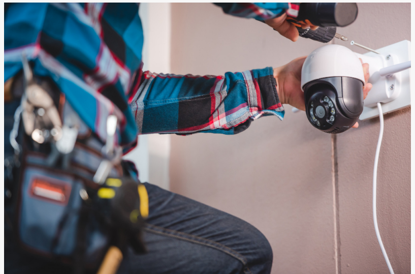
CCTV installation with World Guardian technicians. Installation such as Wifi ip camera Concept: wireless IP camera
