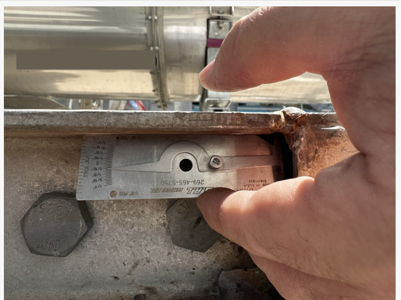
V-WAC Gauge use to check undercut depth on a fullpen CJP AWS D1.1 visual inspection.
